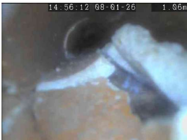
UTPX_60685376-5ae1-4ae4-83d2-2ea7bcbe5f80_20260114_111204_098.jpg, 00:00:14, 1.06 m Broken pipe from 12 o'clock to 12 o'clock
