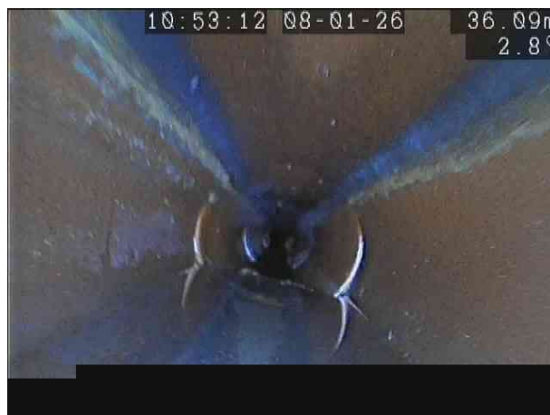
S11X_78b2ec09-74c1-4bdc-9ab7-4dcf4bfc1edf_20260113_13801_547.jpg, 00:02:24, 36.24 m Settled deposits, coarse, 10% cross-sectional area loss
