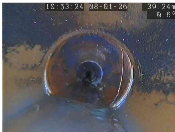
S11X_653b3242-1829-473c-8dc0-a8582c7b2bad_20260113_133827_063.jpg, 00:02:36, 39.24 m Crack, circumferential at joint from 2 o'clock to 5 o'clock
