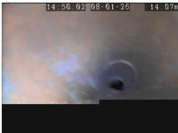
UTPX_7b4baf4e-c8c3-4b1d-b022-2813a2cdd4bd_20260114_105323_879.jpg, 00:00:58, 14.07 m Joint displaced, medium
