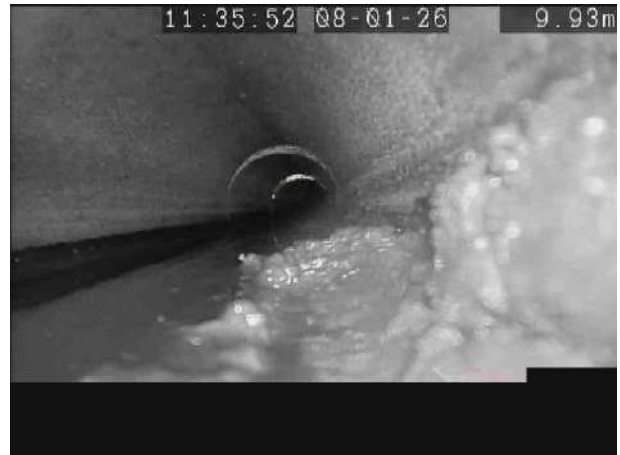
UTPX_b4e2d67c-99ba-4679-9dbe-1ac11ad0f180_20260113_143523_670.jpg, 00:01:22, 9.93 m Settled deposits, fine, 20% cross-sectional area loss
