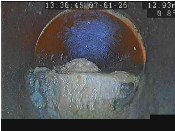
F8X_84287667-c391-46db-8b65-e1f2f57a874d_20260113_10 1457_371.jpg, 00:01:03, 12.92 m Settled deposits, hard or compacted at joint, 30% cross-sectional area loss
