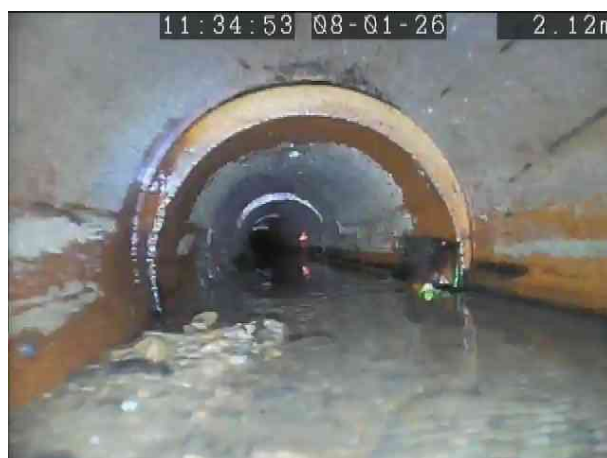
UTPX_a2529226-ab90-4ce5-8443-b7ab9433e7bc_20260113_143304_959.jpg, 00:00:23, 2.24 m Joint displaced, medium
