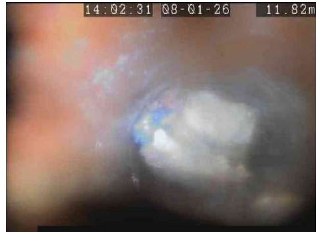
UTPX_ab483161-6365-42ac-83cb-71230abc8909_20260113_163337_861.jpg, 00:00:53, 11.82 m Settled deposits, other, 90% cross-sectional area loss, Debris
