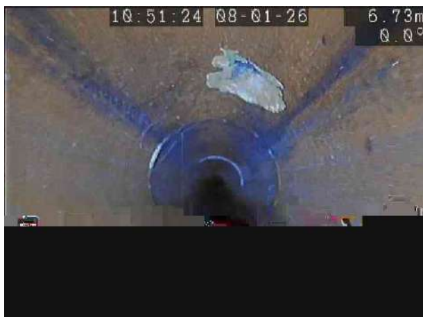
S11X_a5ae82dc-8f31-4991-9271-556768b7a2e0_20260113_133702_749.jpg, 00:00:36, 6.79 m Hole in drain or sewer from 12 o'clock to 1 o'clock
