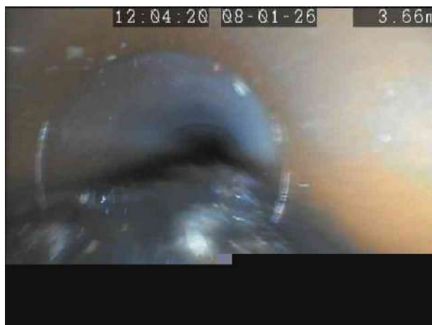
S5X_6ada8f25-3e82-4602-b9c5-5f818bca0afc_20260113_155356_917.jpg, 00:00:11, 0.47 m Settled deposits, coarse, 15% cross-sectional area loss, start
