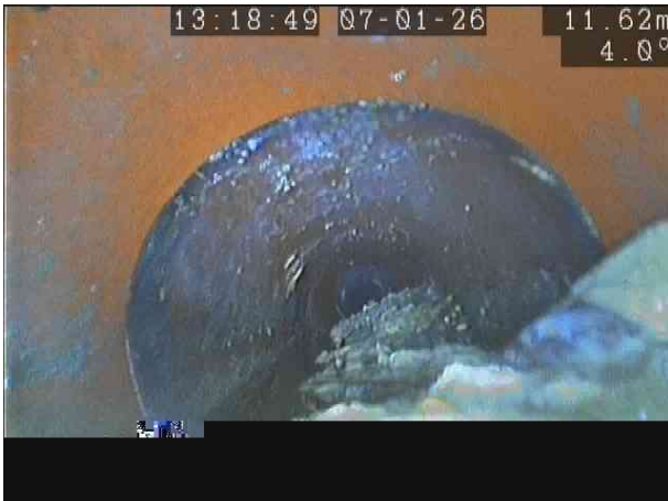
F8X_9d3736a9-4645-4c38-9a23-6f34a04f16f3_20260113_10 1302_611.jpg, 00:01:07, 11.62 m Settled deposits, hard or compacted, 25% cross-sectional area loss
