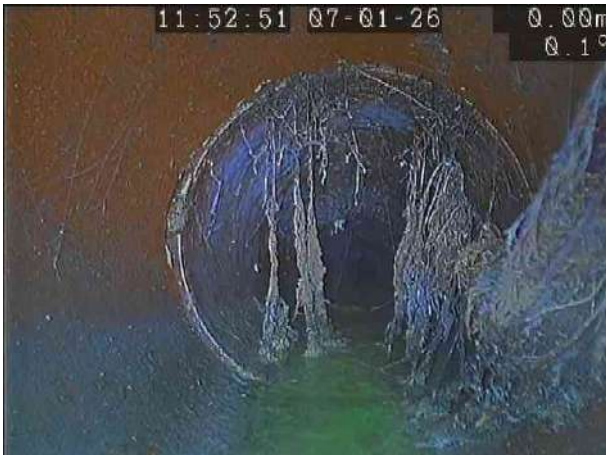
F7X_a7617a19-1f64-4698-bac4-3a5d2f551734_20260112_165335_651.jpg, 00:00:09, 0.01 m Roots, mass at joint, 15% cross-sectional area loss
