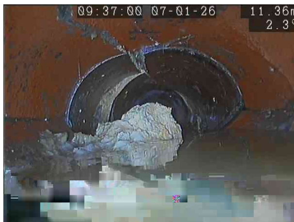
F1X_5838b374-6a7a-4296-a643-91c1efd343d9_20260112_151645_770.jpg, 00:01:11, 11.20 m Broken pipe from 8 o'clock to 5 o'clock
