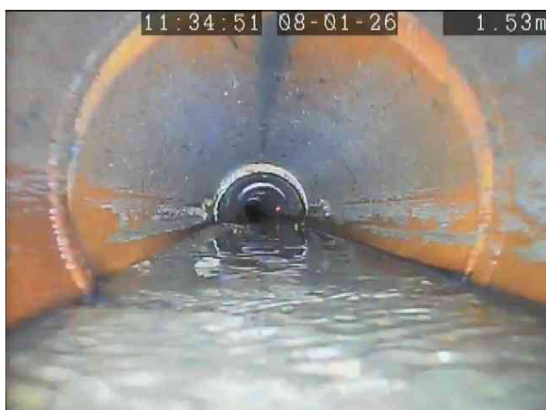
UTPX_9152fd47-bde0-450d-a431-ff0f6197922a_20260113_143244_914.jpg, 00:00:21, 1.65 m Settled deposits, fine, 10% cross-sectional area loss
