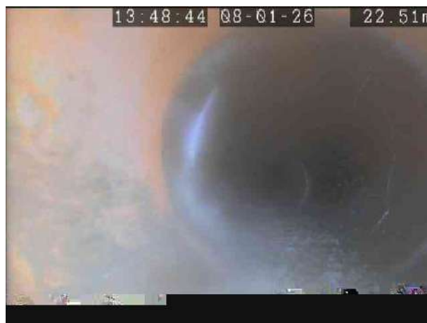
MH DX_cb897b6e-0abc-422c-896a-ad59f3276434_20260113_16 2328_795.jpg, 00:01:19, 22.51 m Crack, circumferential from 8 o'clock to 4 o'clock
