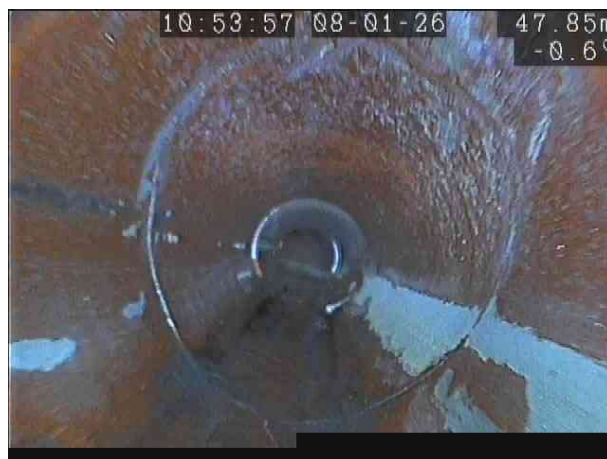
S11X_aabb6734-aea7-4a7f-9b52-c7fee8de099a_20260113_133857_576.jpg, 00:03:09, 47.85 m Crack, circumferential from 4 o'clock to 10 o'clock
