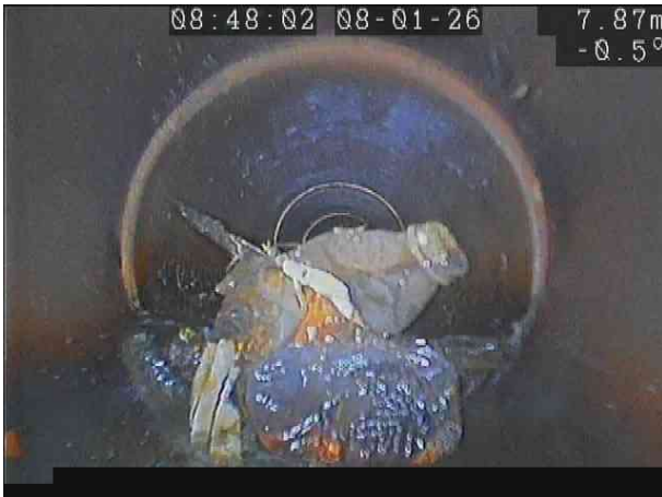
S15X_a3e62ddc-09b3-4e1a-94f0-23bec06ba4d_20260113_121017_307.jpg, 00:00:38, 7.97 m Settled deposits, other at joint, 35% cross-sectional area loss, Debris/ plastic bottle
