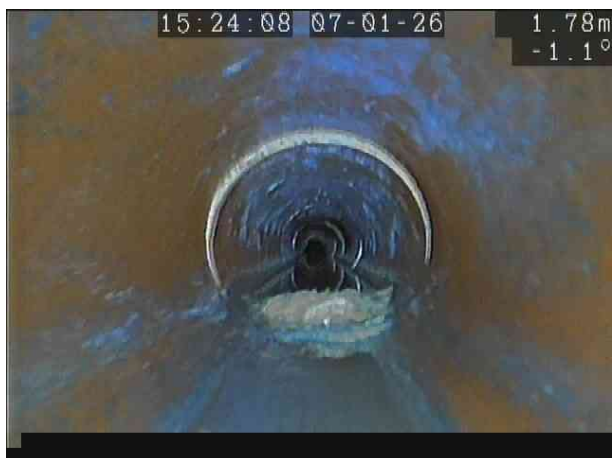
F10X_88d41539-e7ef-4e7b-9146-b98c0a2fe256_20260113_1 13814_053.jpg, 00:00:20, 1.95 m Settled deposits, coarse, 10% cross-sectional area loss
