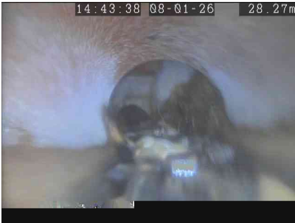
F16X_2f838f91-d5d2-4b1d-8e11-553e0241beff_20260114_10 2301_556.jpg, 00:01:53, 28.51 m Settled deposits, coarse, 15% cross-sectional area loss
