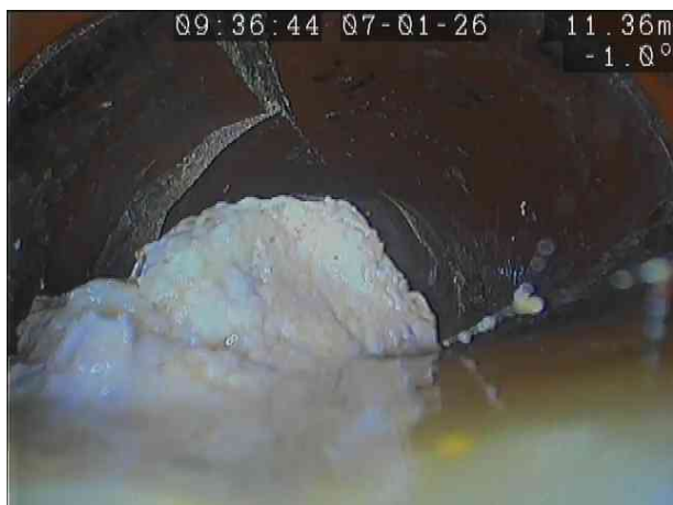
F1X_410dbf36-2f06-44dd-a2a4-ce88e90eca63_20260112_151726_322.jpg, 00:01:27, 11.35 m Settled deposits, other, 25% cross-sectional area loss, Build up of deposits/ tissue
