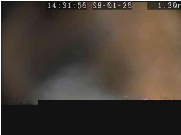
UTPX_f0da44cc-15db-4b21-8a3d-ce97a95c2731_20260113_163301_246.jpg, 00:00:18, 1.41 m Settled deposits, hard or compacted, 10% cross-sectional area loss
