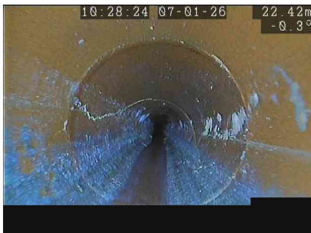
F4X_03cf1129-bd24-41dc-97ae-39b5bc84fe72_20260112_16 0921_010.jpg, 00:01:48, 22.60 m Cracks, spiral from 9 o'clock to 3 o'clock
