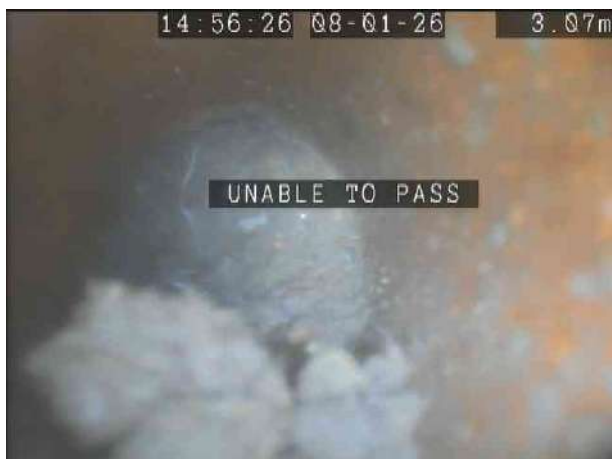
UTPX_049c198c-9e2a-453d-b634-c4a30d34fb20_20260114_111259_330.jpg, 00:00:24, 3.07 m Settled deposits, other, 100% cross-sectional area loss, Debris
