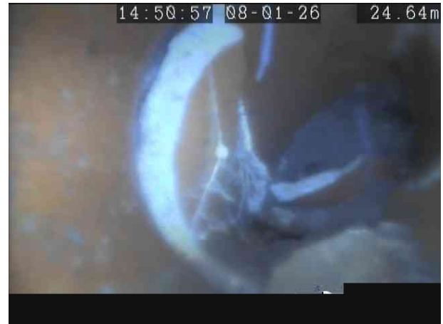
UTPX_0f935942-1346-4250-94bf-d19fa8eb3824_20260114_1 10939_005.jpg, 00:01:53, 24.64 m Collapsed drain or sewer
