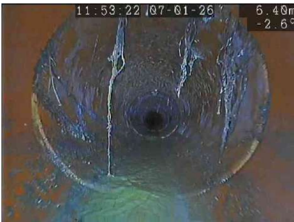
F7X_f6897426-25d9-4469-9ce7-0d661897e67b_20260112_165704_010.jpg, 00:00:39, 6.50 m Roots, fine at joint
