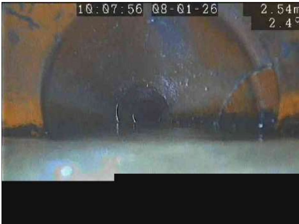
S14X_1265df48-cd84-4abf-a135-6a8a5ebc4b1e_20260113_130230_779.jpg, 00:00:19, 2.54 m Fracture, circumferential at joint from 3 o'clock to 5 o'clock
