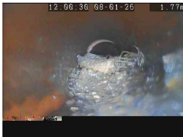
UTPX_d5d5ac0d-9251-43e8-9573-b3638ff8d5a3_20260113_151810_229.jpg, 00:00:39, 1.53 m Settled deposits, hard or compacted, 30% cross-sectional area loss
