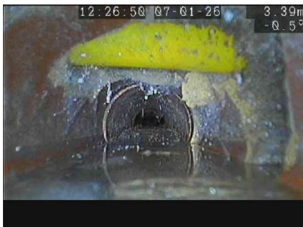
UTPX_068653f2-f03b-49b8-a3ec-4a80fe382551_20260113_100413_502.jpg, 00:00:26, 3.39 m Hole in drain or sewer from 11 o'clock to 4 o'clock
