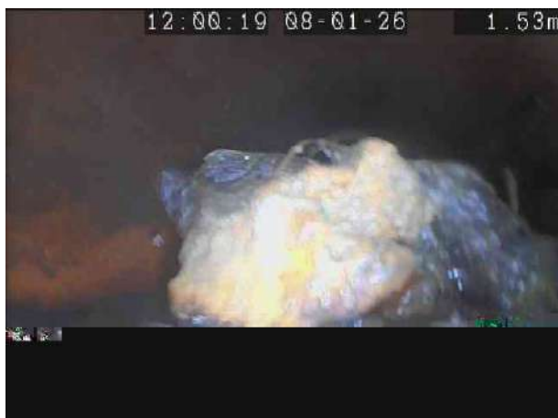
UTPX_04fdff69-ce8d-4378-8e83-d3c481d01a17_20260113_151715_952.jpg, 00:00:25, 1.41 m Settled deposits, coarse, 20% cross-sectional area loss
