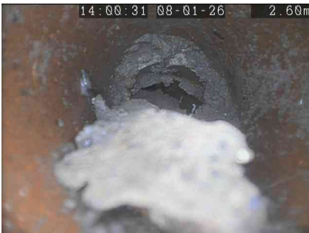
UTPX_ed5cc436-2644-4cf9-9df2-8e11c174298c_20260113_163043_417.jpg, 00:00:28, 2.60 m Settled deposits, coarse, 30% cross-sectional area loss
