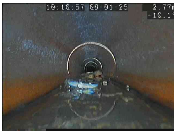
S13X_52196364-0c1f-4e05-ac79-6a31fdc48fa8_20260113_1340_009.jpg, 00:00:22, 2.89 m Settled deposits, other, 5% cross-sectional area loss, Debris
