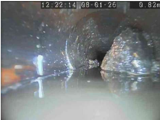
S4X_c187923e-faa9-489e-92a3-b0c3965ce571_20260113_155921_341.jpg, 00:00:17, 0.82 m Settled deposits, other, 40% cross-sectional area loss, Stone, being pushed down line by camera
