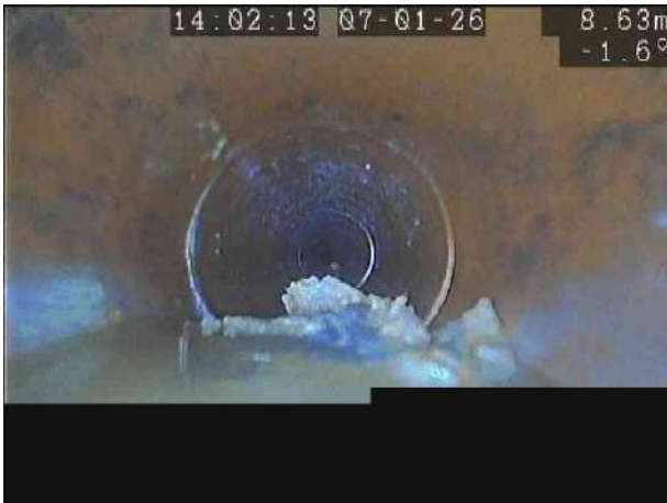
F10X_2241bef5-0425-4b50-a731-9f2defc135dc_20260113_11 1929_897.jpg, 00:01:08, 8.63 m Settled deposits, coarse, 20% cross-sectional area loss
