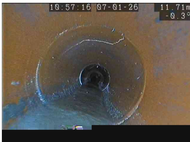
F5X_17059ce4-4398-4c52-ba4e-9d7219542f39_20260112_162807_562.jpg, 00:00:56, 11.79 m Crack, circumferential at joint from 10 o'clock to 1 o'clock
