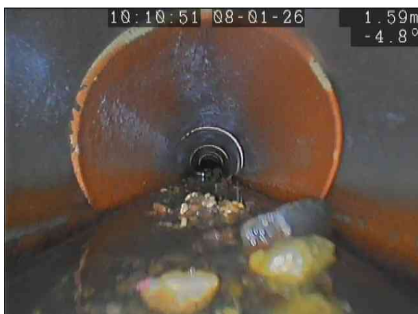
S13X_0c0f28c0-cfb1-46c2-beb2-973ad5f70520_20260113_1311_021.jpg, 00:00:16, 1.68 m Settled deposits, coarse, 10% cross-sectional area loss
