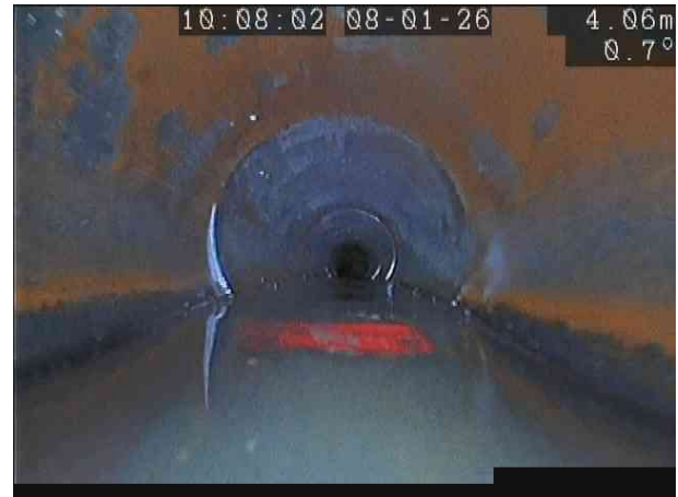
S14X_aeea9044-2881-4b75-9df7-7db3bc777343_20260113_130218_960.jpg, 00:00:26, 4.24 m Settled deposits, other, 10% cross-sectional area loss, Debris
