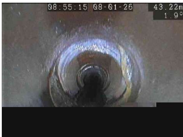
S16X_a20f60a6-8377-404d-8f5c-93dc0efe2f6d_20260113_12 4859_558.jpg, 00:02:15, 43.35 m Settled deposits, hard or compacted at joint, 5% cross-sectional area loss
