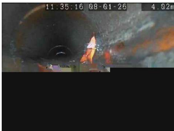
UTPX_28e012c4-69e8-44f5-a731-faab1eb67e50_20260113_143405_048.jpg, 00:00:45, 4.02 m Settled deposits, fine, 10% cross-sectional area loss
