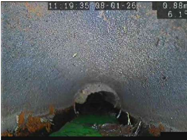
S8X_5068fb8f-3040-4de8-9fec-f176815e66c3_20260113_134 602_467.jpg, 00:00:15, 0.88 m Settled deposits, hard or compacted, 15% cross-sectional area loss
