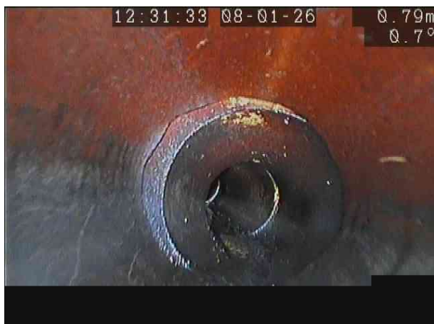
S1X_5cbb6176-5e30-49f6-9dc7-2510361e1031_20260113_160632_197.jpg, 00:00:09, 0.87 m Joint displaced, medium
