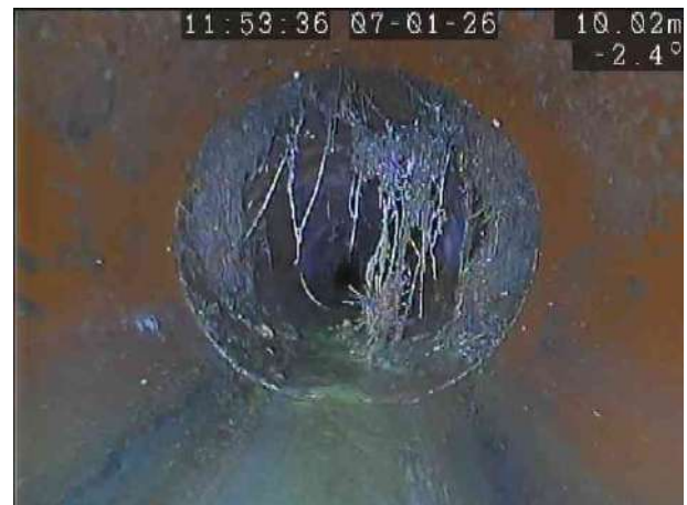
F7X_16e2086c-53f8-490f-a301-c7bc64bf3d63_20260112_165733_648.jpg, 00:00:54, 10.02 m Roots, mass at joint, 10% cross-sectional area loss
