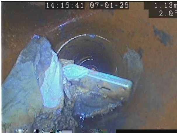
UTPX_2f9e182f-578a-47a9-88cd-600bebfa87a2_20260113_1 12326_332.jpg, 00:00:21, 1.17 m Settled deposits, other, 50% cross-sectional area loss, Debris
