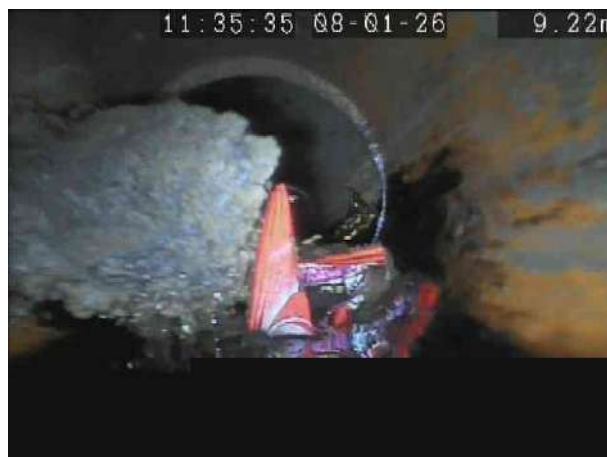
UTPX_86c9f49b-461c-467a-a9d2-2ad092566d19_20260113_143438_824.jpg, 00:01:05, 9.22 m Settled deposits, hard or compacted, 30% cross-sectional area loss
