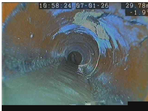
F5X_3cfdc30e-0c9d-4ad8-b902-7c392805fc84_20260112_163217_809.jpg, 00:02:05, 29.78 m Hole in drain or sewer from 12 o'clock to 1 o'clock
