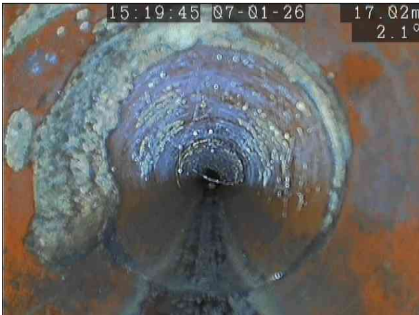
UTPX_f1ed41dd-33af-4494-9a98-af8f18476f67_20260113_11 3448_566.jpg, 00:01:38, 17.00 m Settled deposits, hard or compacted at joint, 10% cross-sectional area loss
