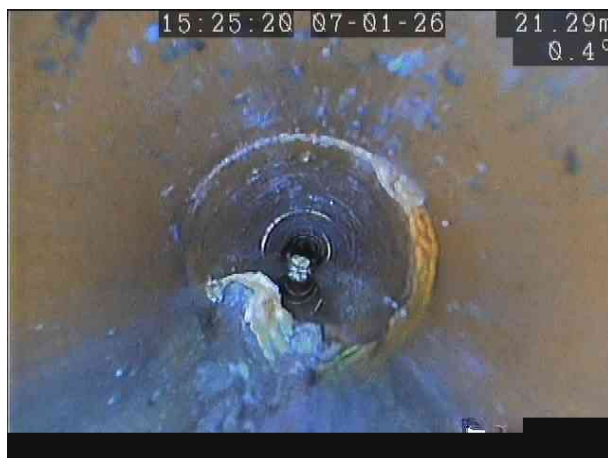
F10X_03a1ed7f-639c-4285-9c20-3d476a801cbd_20260113_1 14036_478.jpg, 00:01:31, 21.29 m Settled deposits, coarse, 15% cross-sectional area loss
