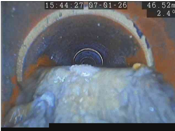
F14X_1960642a-ba62-4ee5-b12e-33e46168597f_20260113_115826_759.jpg, 00:03:34, 46.52 m Settled deposits, other at joint, 55% cross-sectional area loss, Debris/ concrete/ tissue build up
