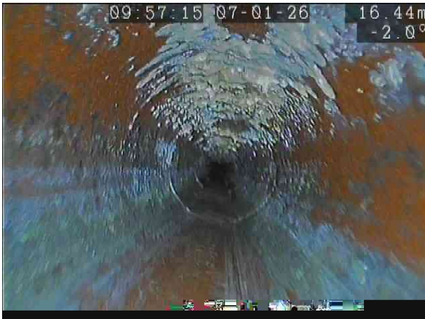
F2X_6ea8c725-9d15-4891-b02f-e35e0dad0f40_20260112_153618_517.jpg, 00:01:14, 16.44 m Attached deposits, grease from 11 o'clock to 1 o'clock, 5% cross-sectional area loss
