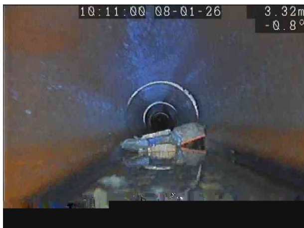
S13X_284dbb6e-bbb9-4e68-9bf0-0350a6dba110_20260113_131353_777.jpg, 00:00:25, 3.46 m Settled deposits, other, 20% cross-sectional area loss, Debris
