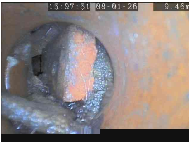
UTPX_85b4a09b-db1d-44b5-8b91-6d594213f920_20260114_111750_863.jpg, 00:00:35, 9.46 m Settled deposits, other, 90% cross-sectional area loss, Debris
