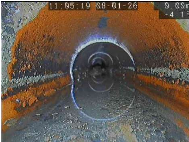
S8X_c7d417f2-d3ed-491a-adc4-e6cd4da9f15a_20260113_134027_752.jpg, 00:00:08, 0.01 m Settled deposits, hard or compacted, 5% cross-sectional area loss, start
