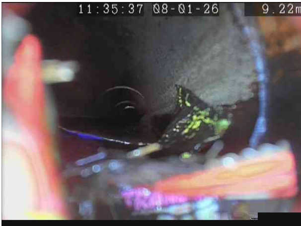
UTPX_2497b55d-662b-4426-9aa4-05de989d99aa_20260113_143450_921.jpg, 00:01:06, 9.46 m Settled deposits, other, 15% cross-sectional area loss, Debris
