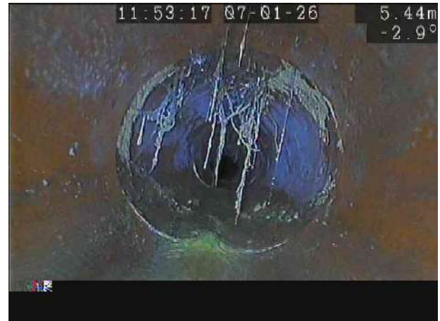
F7X_3d5f8c96-7b21-4198-9444-d0aeda95a7ea_20260112_165653_177.jpg, 00:00:35, 5.52 m Roots, fine at joint
