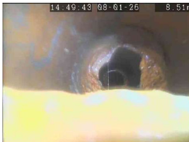
UTPX_8bb7cd00-efc-41fb-a15a-5ea06e7c3178_20260114_103230_866.jpg, 00:00:40, 8.75 m Settled deposits, hard or compacted at joint, 20% cross-sectional area loss
