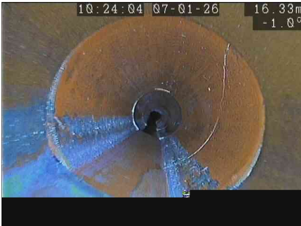
F3X_d4a1069f-cfc8-4e9f-a40a-843b956b0bde_20260112_155 647_153.jpg, 00:01:19, 16.42 m Crack, circumferential from 2 o'clock to 5 o'clock
