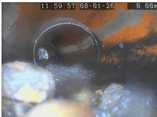
UTPX_0ad9181f-6c8b-47ef-a044-a9811f1b18ec_20260113_151543_568.jpg, 00:00:07, 0.01 m Settled deposits, coarse, 10% cross-sectional area loss
