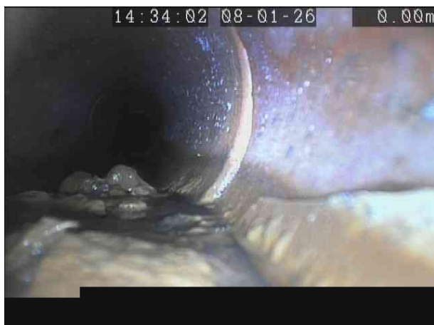
F15X_e000a593-2e50-419e-b63e-41e633074d94_20260113_165104_531.jpg, 00:00:08, 0.01 m Settled deposits, coarse, 10% cross-sectional area loss
