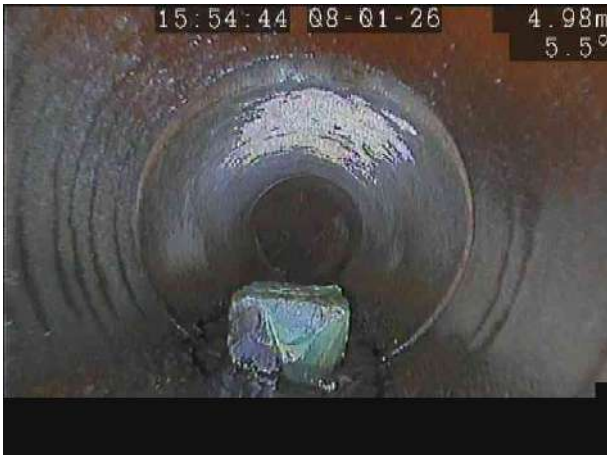
S19X_ed8da343-b3db-47a3-9643-4201a8f57023_20260114_114237_494.jpg, 00:00:27, 4.98 m Settled deposits, coarse, 15% cross-sectional area loss
