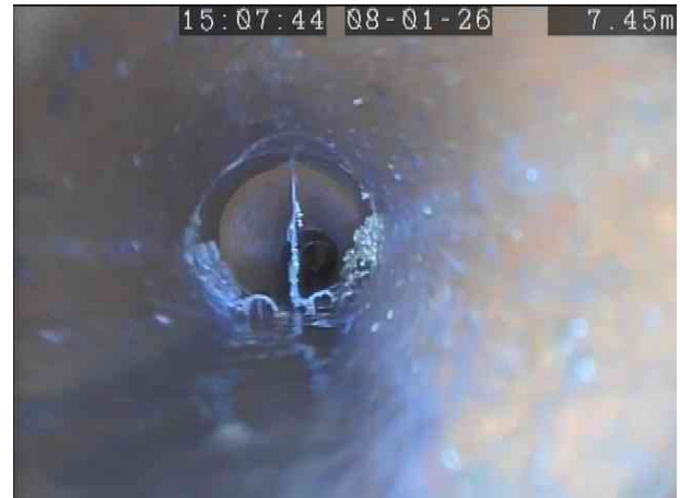
UTPX_d8244e51-3385-48a3-b232-4742af6de5db_20260114_111646_958.jpg, 00:00:27, 7.57 m Roots, fine at joint
