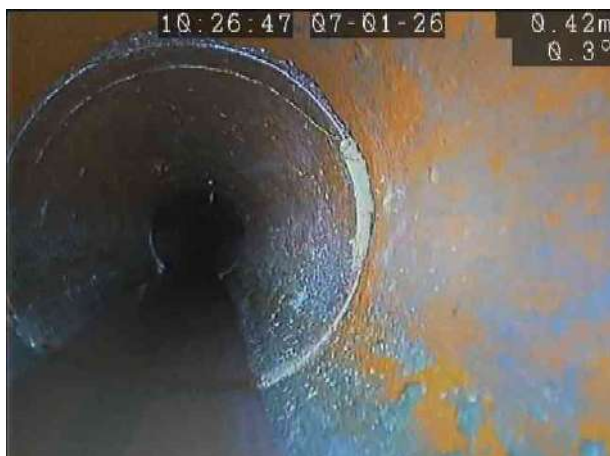
F4X_a9e5a6e2-4a96-432f-8085-0c3a392ff9b0_20260112_16 0750_892.jpg, 00:00:10, 0.46 m Crack, circumferential at joint from 9 o'clock to 2 o'clock
