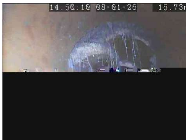
UTPX_e4a97761-bf7c-435b-a29f-8b08a638f5a0_20260114_105417_165.jpg, 00:01:06, 15.84 m Broken pipe from 12 o'clock to 12 o'clock
