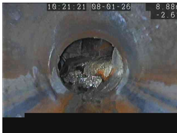
S12X_49f3b57a-a9ff-4c89-90a3-f8d0d7894cd5_20260113_131950_414.jpg, 00:01:04, 9.03 m Crack, circumferential from 9 o'clock to 10 o'clock
