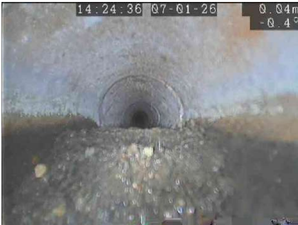
F12X_90689cb1-e125-4233-8793-0bcb1e314596_20260113_112434_945.jpg, 00:00:10, 0.10 m Settled deposits, fine, 20% cross-sectional area loss
