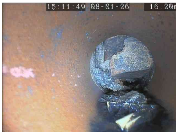
UTPX_5e684cd7-e4e7-440e-8c9b-5b91ab39ce6e_20260114_112940_235.jpg, 00:00:46, 16.20 m Settled deposits, other, 80% cross-sectional area loss, Debris
