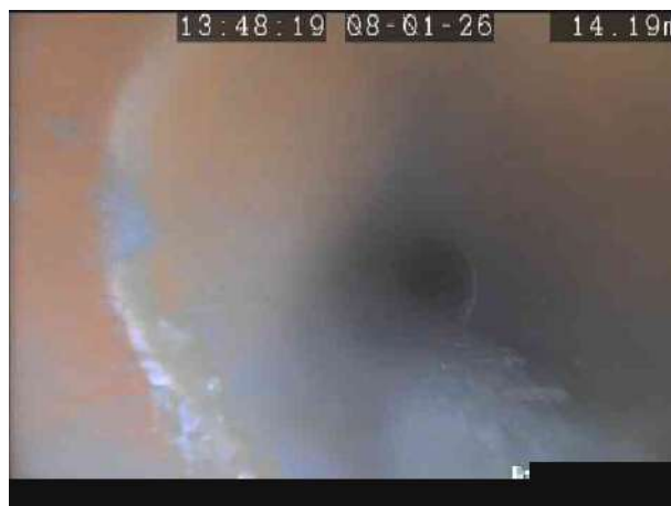
MH DX_4d03ee10-df75-476a-8073-63a1b75a21cd_20260113_16 2241_781.jpg, 00:00:55, 14.43 m Settled deposits, hard or compacted, 5% cross-sectional area loss
