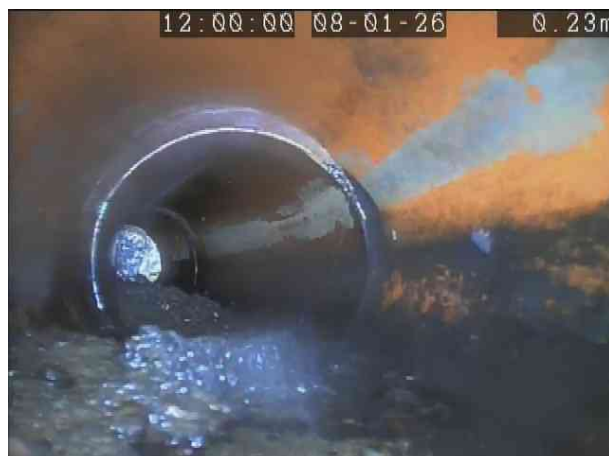
UTPX_a7ab876b-5cf9-45df-ba0d-2c3f9d88bf90_20260113_151629_947.jpg, 00:00:09, 0.05 m Settled deposits, hard or compacted, 10% cross-sectional area loss
