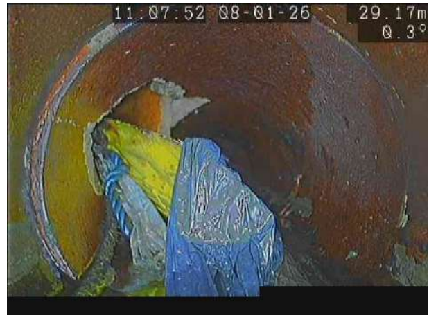
S8X_5000703f-c1d5-4867-86c9-8a02e158d579_20260113_134438_778.jpg, 00:02:40, 29.17 m Settled deposits, other, 30% cross-sectional area loss, Debris
