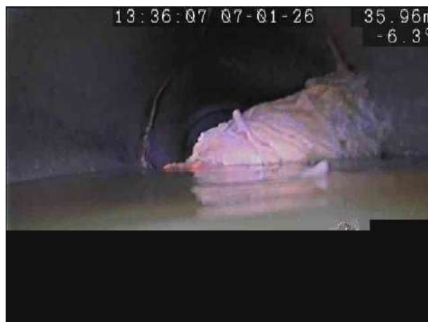
F9X_af65bf37-e4e7-4cdc-a093-bc78bb8aae3f_20260113_103211_161.jpg, 00:02:39, 35.96 m Settled deposits, other, 35% cross-sectional area loss, Debris and tissue build up
