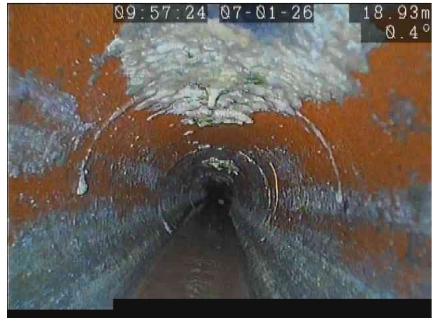
F2X_846ea05a-ec3a-43e2-84c1-b983d22ed349_20260112_153831_818.jpg, 00:01:24, 18.93 m Attached deposits, grease from 11 o'clock to 1 o'clock, 5% cross-sectional area loss
