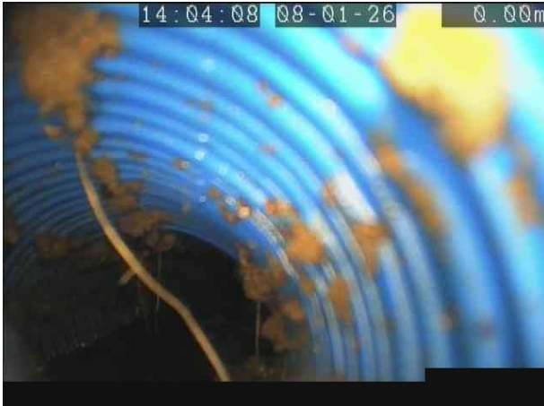
UTPX_2ede97d7-f706-4200-879c-3324adf5b2be_20260113_163638_691.jpg, 00:00:13, 0.05 m Settled deposits, fine, 15% cross-sectional area loss
