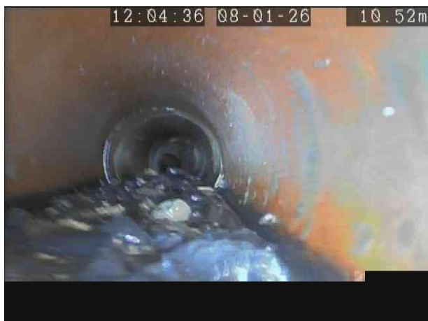
S5X_17eee903-8ff5-46f8-a699-af2aa11c2443_20260113_155422_302.jpg, 00:00:35, 10.88 m Crack, circumferential at joint from 8 o'clock to 2 o'clock
