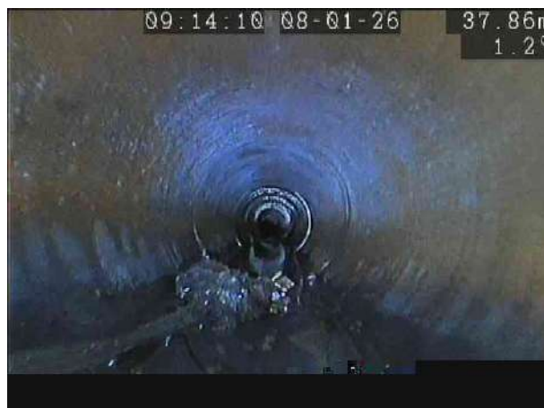
S18X_4f0a740e-0d83-4d53-a602-a755721c1a30_20260113_125806_873.jpg, 00:02:14, 38.03 m Settled deposits, coarse, 5% cross-sectional area loss
