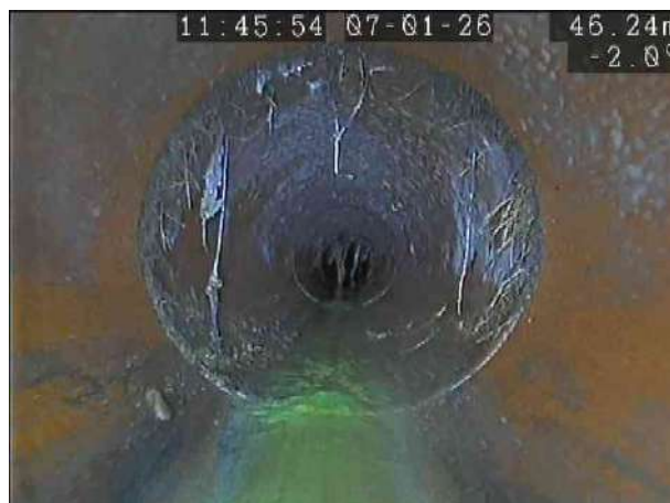
F6X_e61b8769-9f19-422e-b610-2d909e8e712a_20260112_1 64823_396.jpg, 00:03:13, 46.32 m Roots, fine at joint
