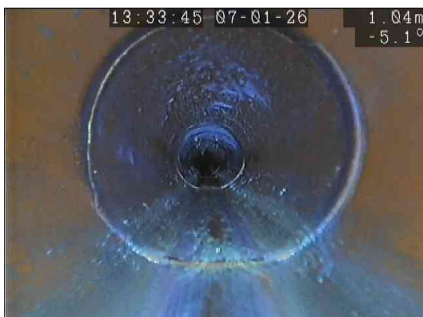
F9X_7a347b84-d681-4ce0-9d2c-b3cefc7ed3d8_20260113_101746_845.jpg, 00:00:16, 1.11 m Crack, circumferential at joint from 8 o'clock to 1 o'clock
