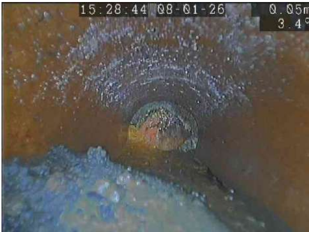
UTPX_b1e6c33d-a59f-43bf-90de-e2c031dc2c8c_20260114_1 13303_394.jpg, 00:00:11, 0.08 m Settled deposits, hard or compacted, 20% cross-sectional area loss
