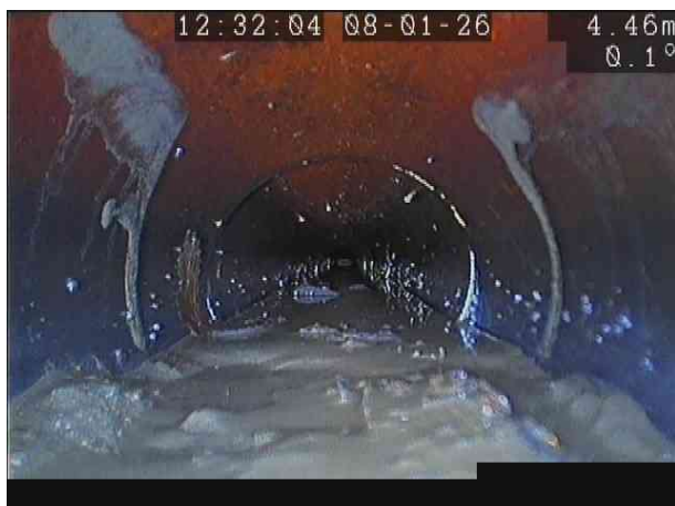
S1X_ff8da6ed-839d-4570-b4ff-7c0343390d01_20260113_160946_324.jpg, 00:00:40, 4.46 m Settled deposits, coarse, 10% cross-sectional area loss
