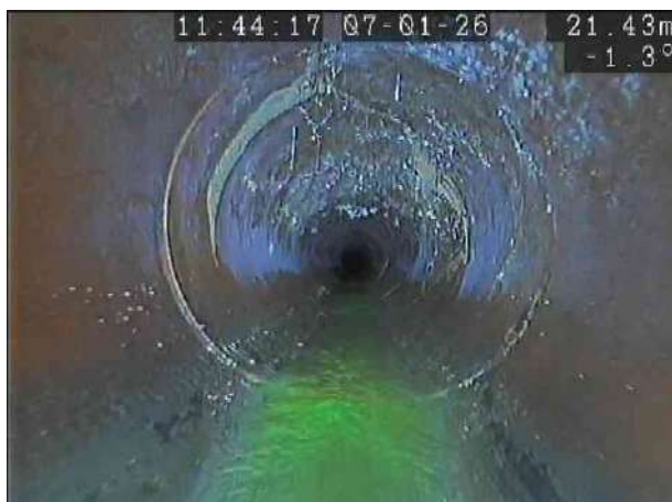
F6X_ac076561-1e8e-471a-937a-8ed1a30195ee_20260112_1 64600_330.jpg, 00:01:36, 21.52 m Fracture, circumferential from 9 o'clock to 2 o'clock
