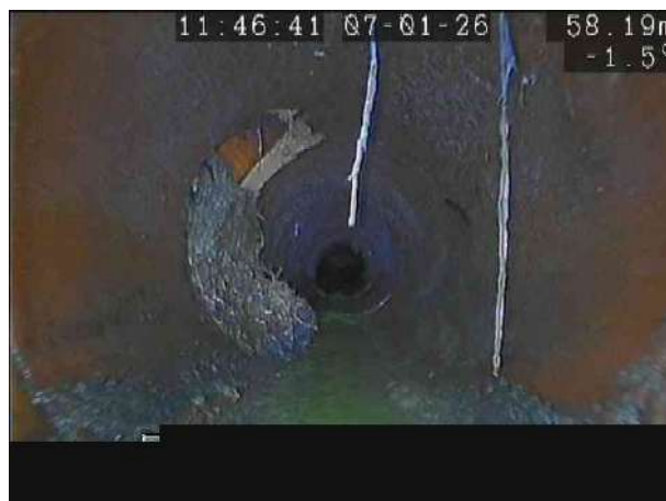
F6X_f55eae9c-39f0-4812-8dcb-4fb0534bb419_20260112_165 048_351.jpg, 00:04:01, 58.34 m Roots, mass, 15% cross-sectional area loss
