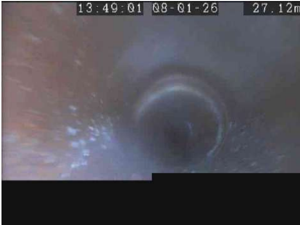
MH DX_423219d4-26d9-43dc-9b9d-a2cc66988e55_20260113_16 2404_296.jpg, 00:01:36, 27.36 m Crack, circumferential from 10 o'clock to 4 o'clock
