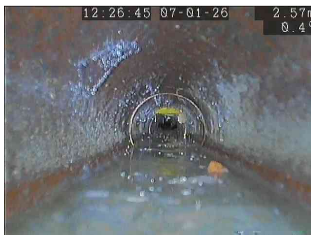
UTPX_c85c12ec-a350-4859-b1b6-14da97e40086_20260113_100354_232.jpg, 00:00:21, 2.68 m Settled deposits, fine, 10% cross-sectional area loss
