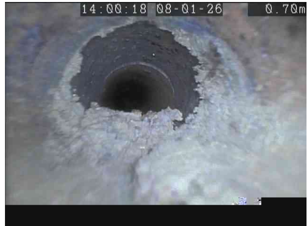
UTPX_60e97b13-af89-4c0c-b4e1-6fdc76e06bcd_20260113_163021_984.jpg, 00:00:15, 0.70 m Settled deposits, coarse, 30% cross-sectional area loss
