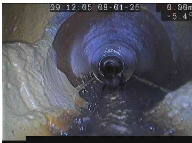
S18X_ce43303f-2ea3-406a-82e7-b5ef4830f96d_20260113_125433_537.jpg, 00:00:09, 0.01 m Settled deposits, hard or compacted, 5% cross-sectional area loss
