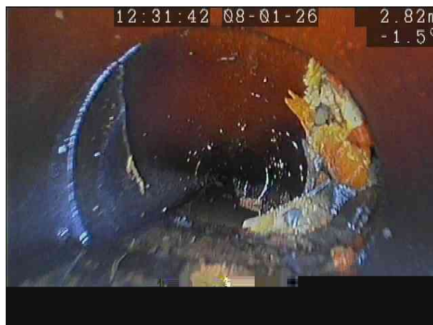
S1X_e6de85a4-e77f-4b3c-874c-8ecab18b4f68_20260113_160719_668.jpg, 00:00:17, 2.82 m Broken pipe from 2 o'clock to 5 o'clock
