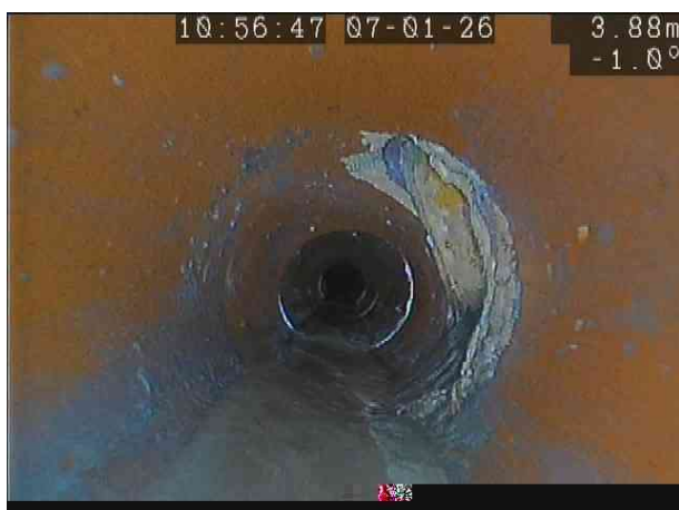
F5X_9deb117e-8430-45e1-b373-aeb99019fc76_20260112_161859_251.jpg, 00:00:28, 3.98 m Hole in drain or sewer at 1 o'clock
