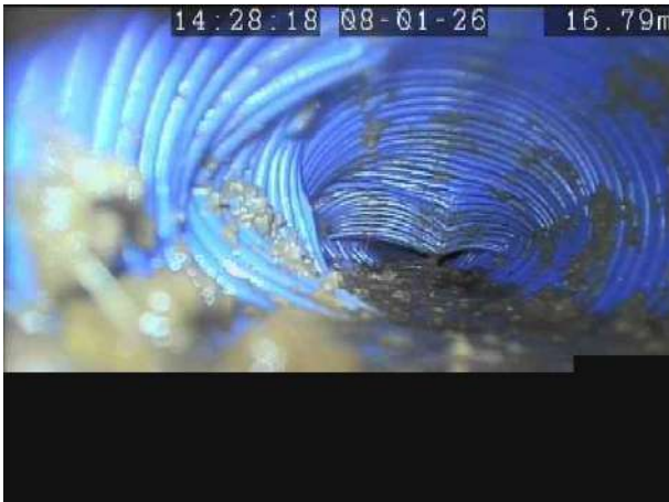
UTPX_97496b37-96e3-48a7-8545-d3d9d306e267_20260113_164418_848.jpg, 00:01:00, 16.91 m Deformed sewer or drain, 20%
