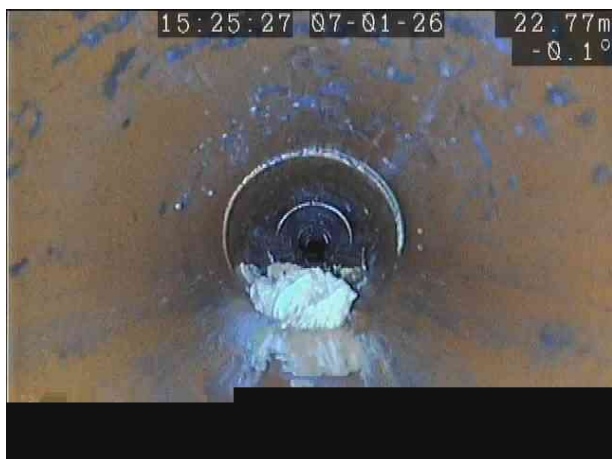
F10X_118fc3c3-2726-4eb2-823e-ee4d103f9151_20260113_1 14053_675.jpg, 00:01:39, 22.93 m Settled deposits, coarse, 15% cross-sectional area loss
