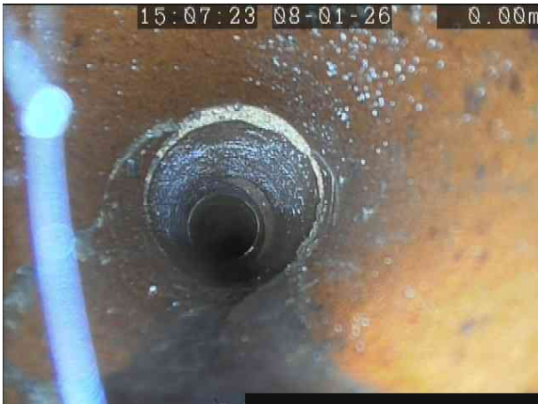
UTPX_00ba62ba-7228-4e3a-ab50-67f647fc064b_20260114_111550_842.jpg, 00:00:07, 0.01 m Fracture, circumferential from 8 o'clock to 5 o'clock
