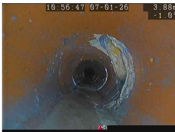
F5X_25828314-b1b5-4540-ac4d-781a8ea3b468_20260112_161740_593.jpg, 00:00:28, 4.06 m Connection other than junction at 2 o'clock, 150mm dia
