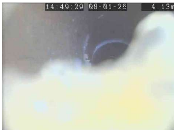
UTPX_c30d5d1f-99a7-486b-8360-744e4e757505_20260114_102854_811.jpg, 00:00:25, 4.25 m Crack, circumferential from 8 o'clock to 1 o'clock
