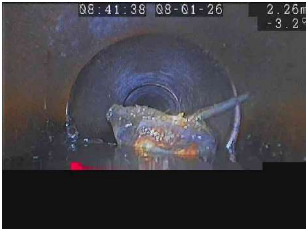
S15X_9e7e1cf3-17cd-4139-ae9a-caa55bf70de6_20260113_1 20110_231.jpg, 00:00:22, 2.26 m Settled deposits, other at joint, 35% cross-sectional area loss, Debris
