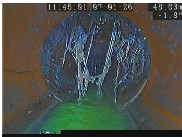
F6X_f7482c4a-01b9-42b9-a6bb-3c2c921dccff_20260112_164 835_226.jpg, 00:03:20, 48.03 m Roots, fine at joint, start
