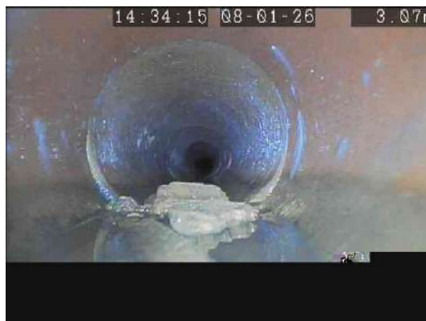
F15X_b6078b49-660c-4a74-9086-629c58fe732a_20260113_165125_038.jpg, 00:00:21, 3.19 m Settled deposits, coarse, 10% cross-sectional area loss
