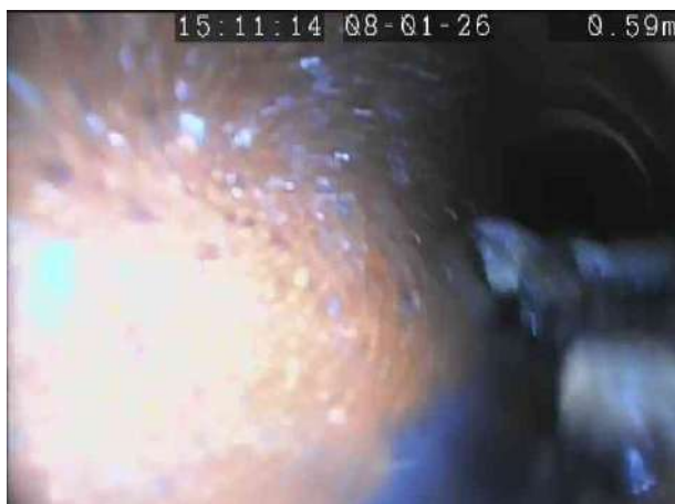
UTPX_ca82abcc-7169-4572-9bf6-a26fde51f873_20260114_112821_891.jpg, 00:00:11, 0.82 m Settled deposits, other, 20% cross-sectional area loss, Debris
