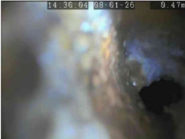
CPX_09ef34f8-83c6-42a6-a88d-1e184cb17af3_20260113_16 4748_242.jpg, 00:00:25, 0.40 m Settled deposits, hard or compacted, 10% cross-sectional area loss
