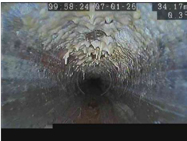
F2X_23e92cbd-ea92-4317-941e-65617c6e4a8e_20260112_153830_698.jpg, 00:02:23, 34.25 m Attached deposits, grease from 10 o'clock to 2 o'clock, 5% cross-sectional area loss, start
