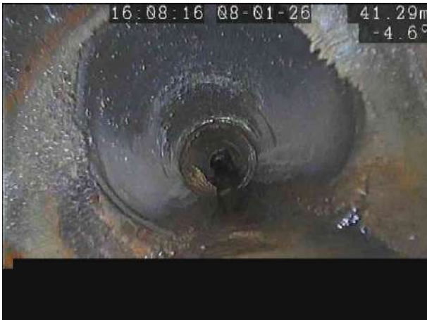
S21X_d07d713c-ec8f-442b-a798-7d4515e179f9_20260114_1 14516_639.jpg, 00:03:02, 41.29 m Settled deposits, hard or compacted at joint, 15% cross-sectional area loss
