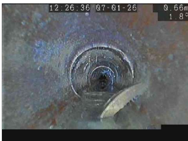
UTPX_a97cce06-e967-4b8a-b8ab-1a1386f52b8b_20260113_100248_391.jpg, 00:00:12, 0.66 m Settled deposits, other, 15% cross-sectional area loss, Debris
