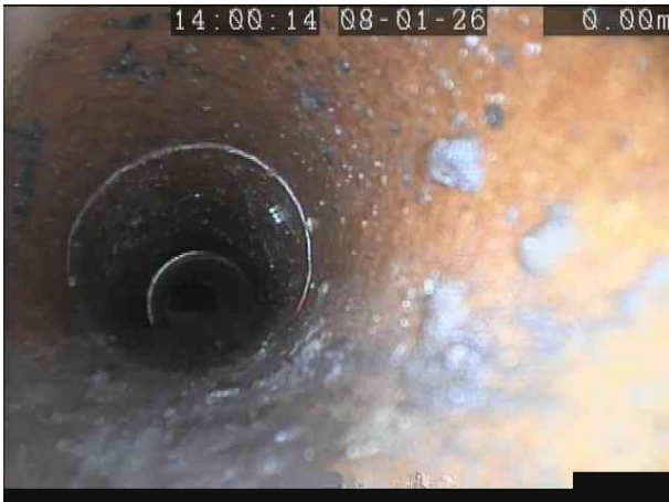
UTPX_c742aa9b-e4e0-4005-b7d6-50032fb3d565_20260113_162922_911.jpg, 00:00:10, 0.05 m Crack, circumferential from 8 o'clock to 4 o'clock
