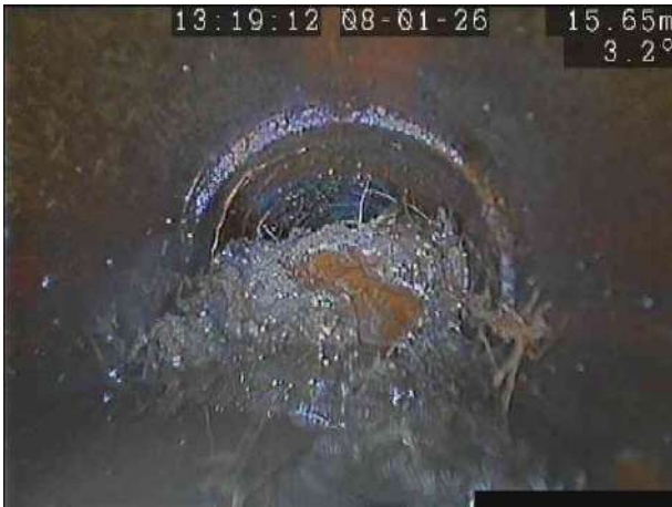
S1X_f4f87085-bfee-4cdb-9785-e85c5f0aa447_20260113_161944_601.jpg, 00:01:29, 15.65 m Settled deposits, other, 70% cross-sectional area loss, Debris
