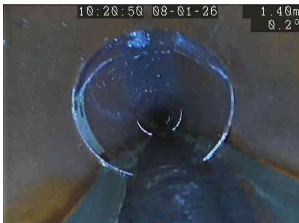
S12X_629ef316-9d30-47f9-8d5b-13e2ddea95e0_20260113_131904_905.jpg, 00:00:33, 1.40 m Crack, circumferential at joint from 9 o'clock to 3 o'clock
