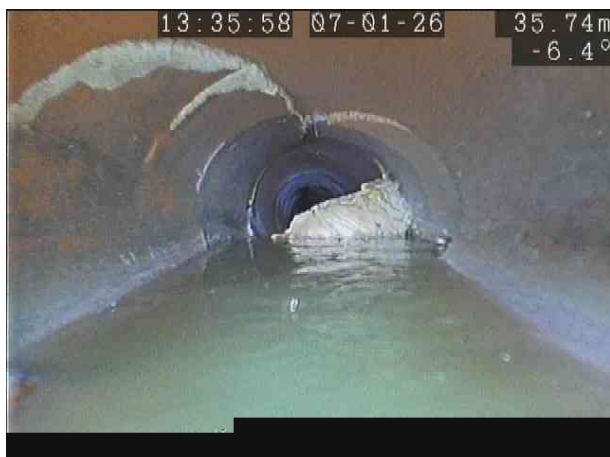
F9X_ac26a8d9-d522-4fa7-8565-7c5dfe7c730_20260113_102022_051.jpg, 00:02:30, 35.85 m Broken pipe from 7 o'clock to 4 o'clock
