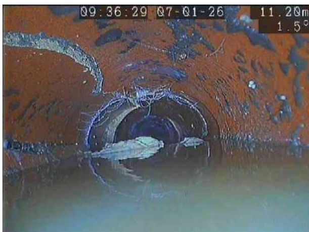
F1X_67b17bf0-8fd4-4490-a28f-ffde36719d92_20260112_151609_193.jpg, 00:01:11, 11.20 m Broken pipe from 8 o'clock to 5 o'clock
