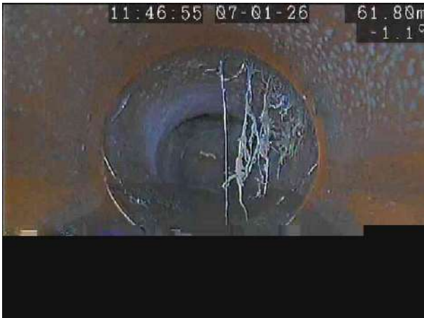
F6X_36172d17-64c7-441e-8fcf-22b09bdb08cb_20260112_16 5135_021.jpg, 00:04:15, 61.89 m Roots, fine at joint
