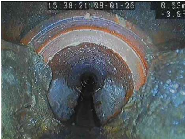
S20X_85b2926b-581d-4bc9-92bc-5925b49397d3_20260114_113431_706.jpg, 00:00:30, 0.53 m Settled deposits, hard or compacted, 15% cross-sectional area loss
