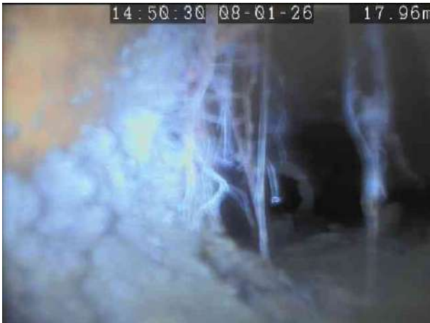
UTPX_dbf57161-392c-4f6e-9c70-0c18ebe38cbd_20260114_1 10852_764.jpg, 00:01:27, 18.09 m Settled deposits, fine, 15% cross-sectional area loss
